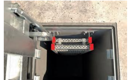
Stormwater overflow tank manholes
